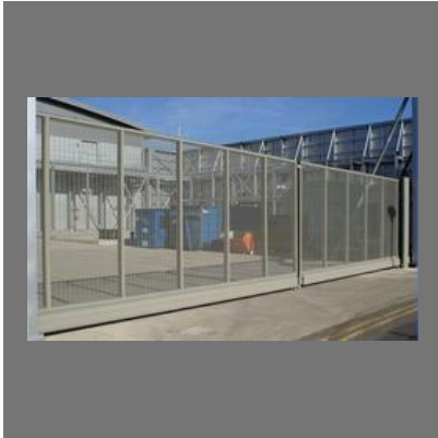
Automatic Electric Sliding Gate
