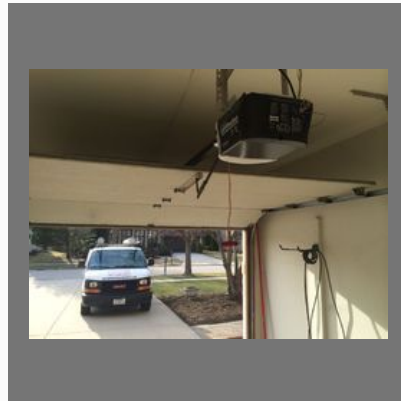
Garage Door Opener
